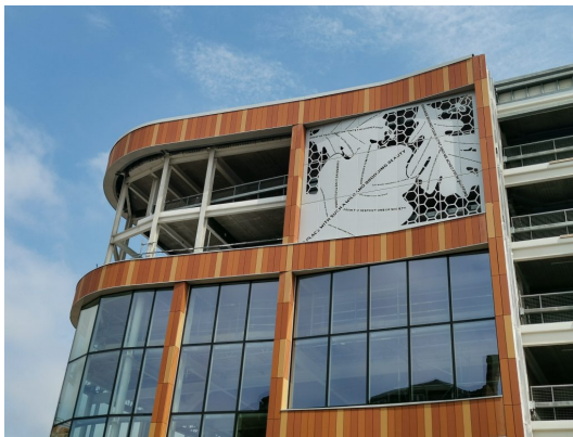
The façade of the new Central Library has just been put in place
