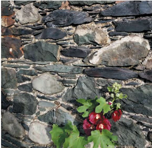
Gathered stone at the front of St Herbert's Social Centre, High Hill, built in 1833. The wall was constructed using a mixture of dark grey to black Skiddaw slate, grey-green Lakeland slate and boulders of rocks from the Borrowdale Volcanic Group
