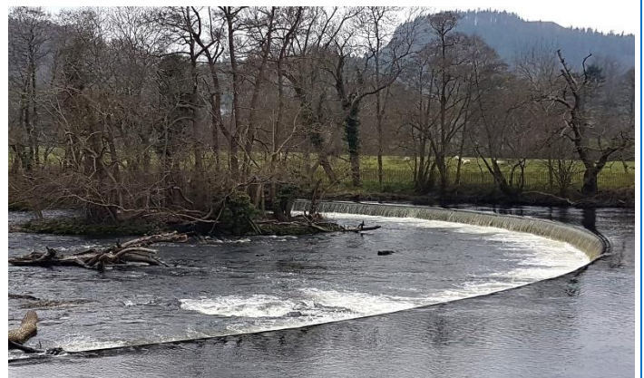
The Horseshoe falls on the River Dee, close to the start of the Llangollen Canal. Photo: Rose Reynolds
