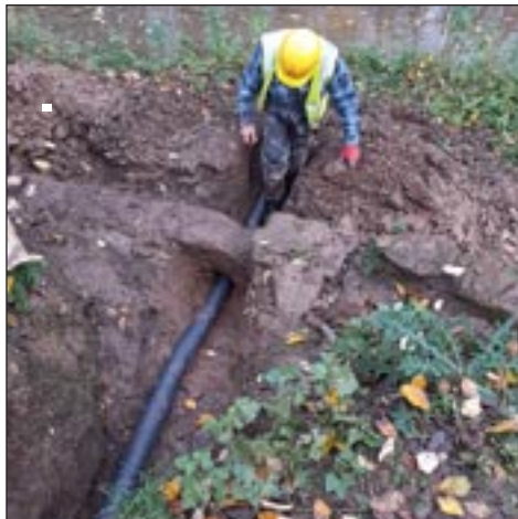
Field drain piped under old retaining wall
