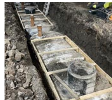
The sewerage installation in the Romney building
