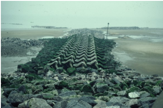
Breakwater designed to be submerged and absorb wave energy.
