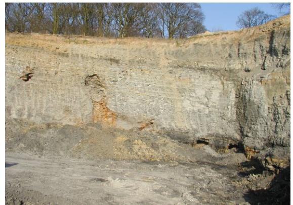
Void migrating upwards in Opencast face – potential serious subsidence.
