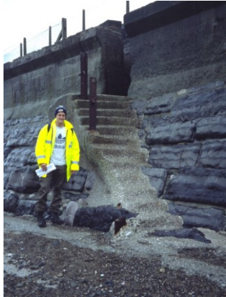
Concrete steps eroded by waves bombarding steps with beach pebbles..
