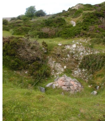
Capped mine shaft. • 36% of Holywell Bypass in Carboniferous Limestone was affected by old workings in mineral veins. • 34 mineshafts capped as part of the road works. • Also 10 reinforced concrete rafts needed to stabilise the upgraded carriageway.
